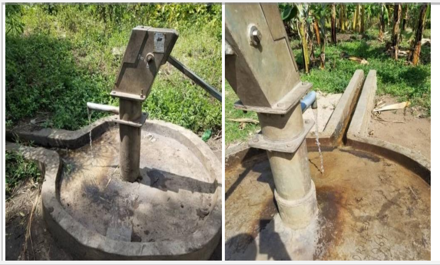
Figure 35: Unfenced borehole of Rusese ward and Nyakahya
