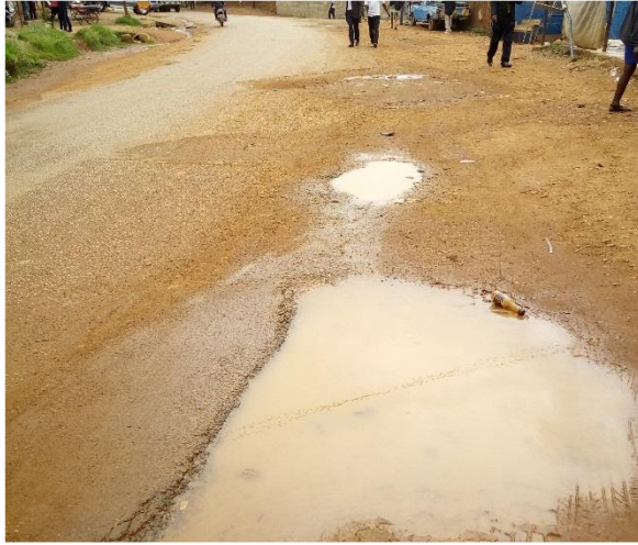
poor current drainage condition and pot holes in the road
