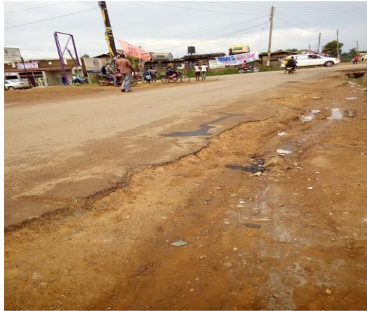
excessive ravelling and of the road
