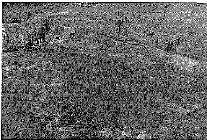
Photograph showing some of the area affected by land slides and covered by stagnant water
